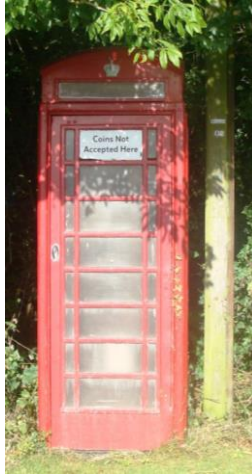
Picture 9. 20th century listed telephone kiosk. Would benefit by undertaking minor repairs and cleansing and if necessary repainting.
