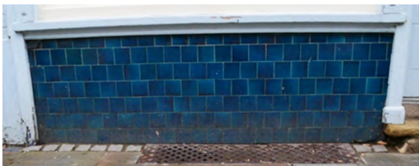
Figure 30 - Glazed blue tiles appropriate to this stallriser.
