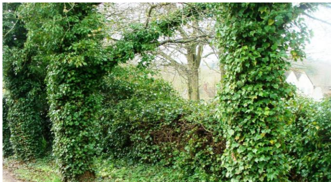
Picture 25. The condition of the eastern boundary of the church boundary wall? is unknown. Suggest explore further and consider implementing any necessary repairs.
