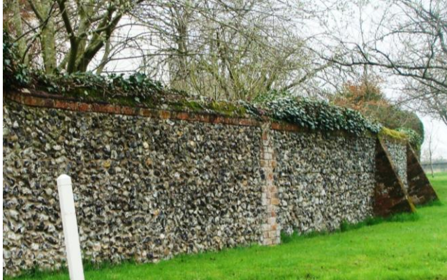
Picture 26. High quality boundary wall to Anstey Hall - a prominent and visually important feature in the street scene.
